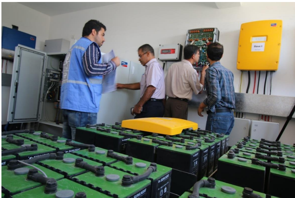
Figure 8: Testing the Installation of Solar System in Al Aqsa Hospital
