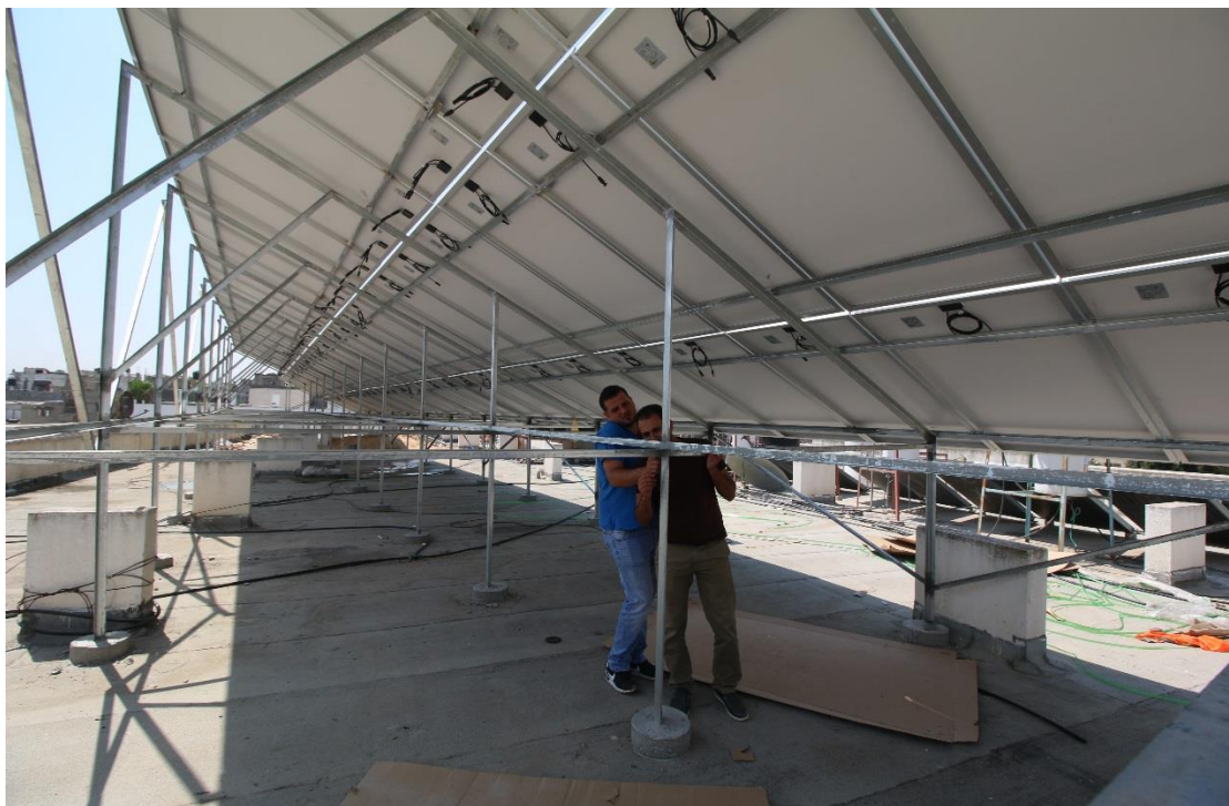
Figure 12: Checking the Steel Structure of the Solar Panels in Beit Hanoun Hospital
