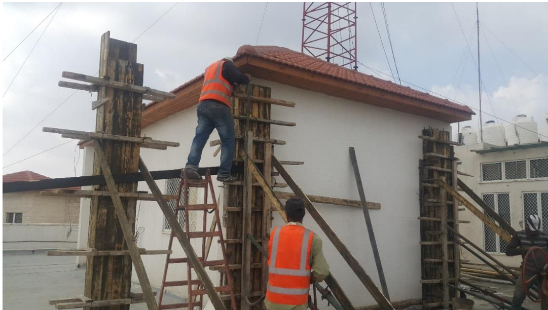
Figure 3: Construction of the Batteries Room on the top of the Indonesian Hospital
