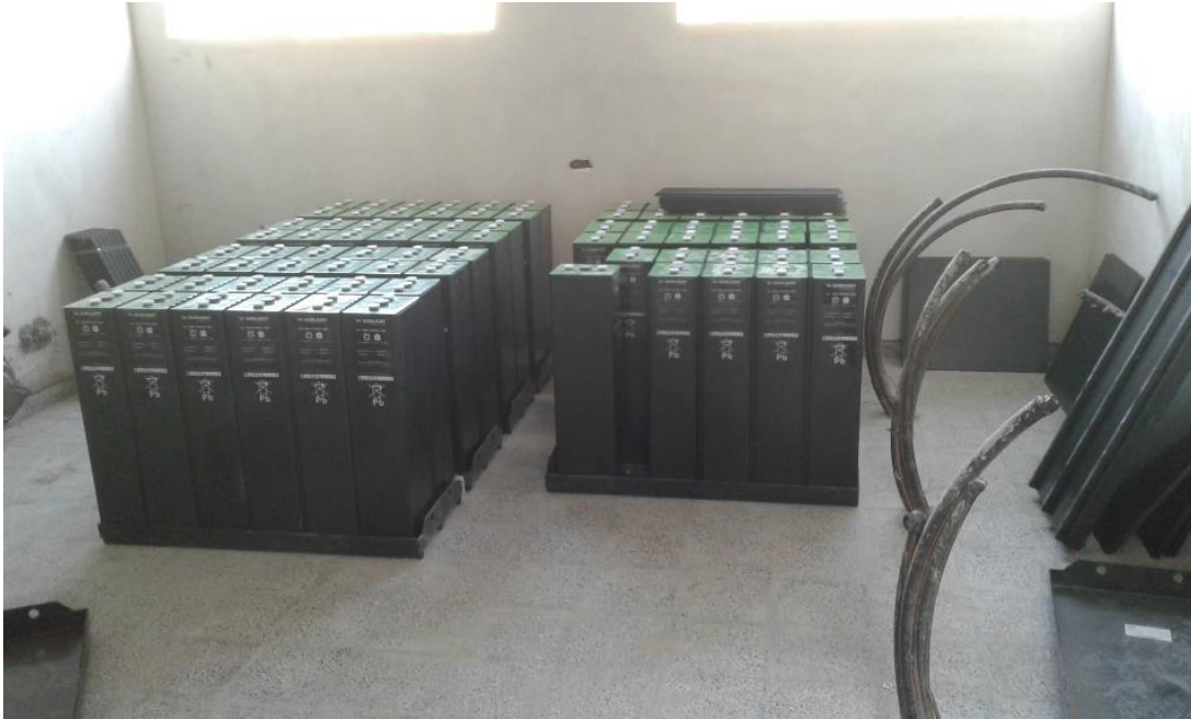
Figure 5: Supplied Batteries in the Batteries Room at Indonesian Hospital
