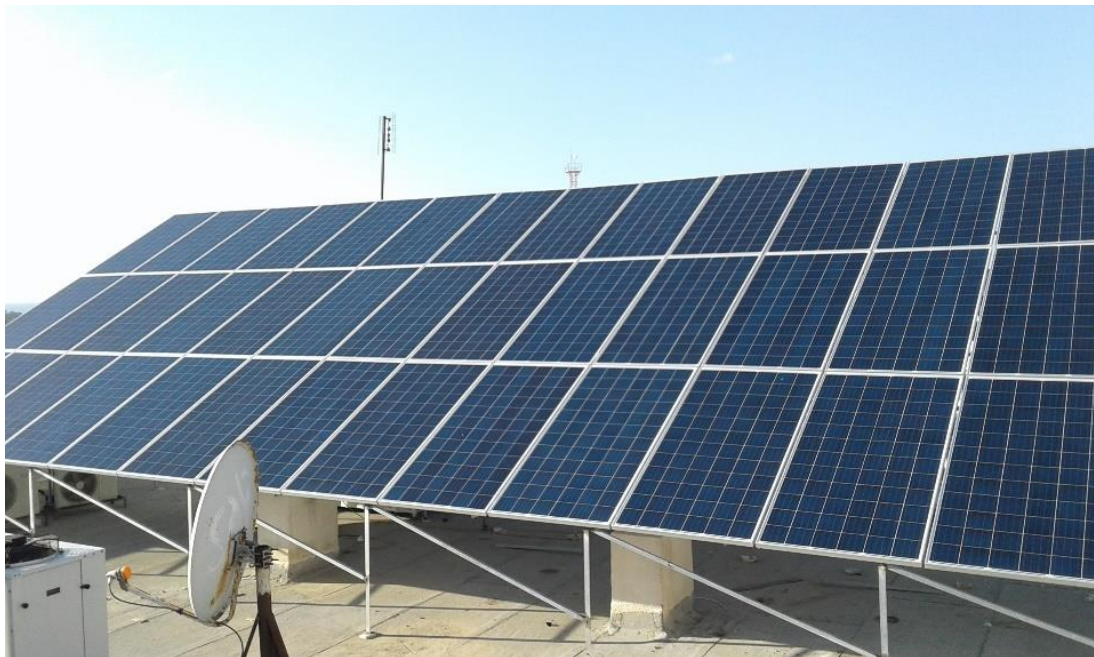
Figure 10: Solar Panels on the top of Al Aqsa Hospital
