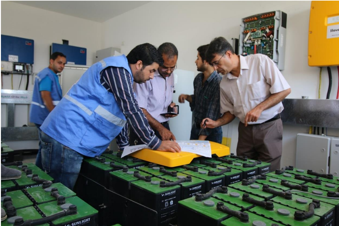
Figure 9: Testing the Installation of Solar System in Al Aqsa Hospital
