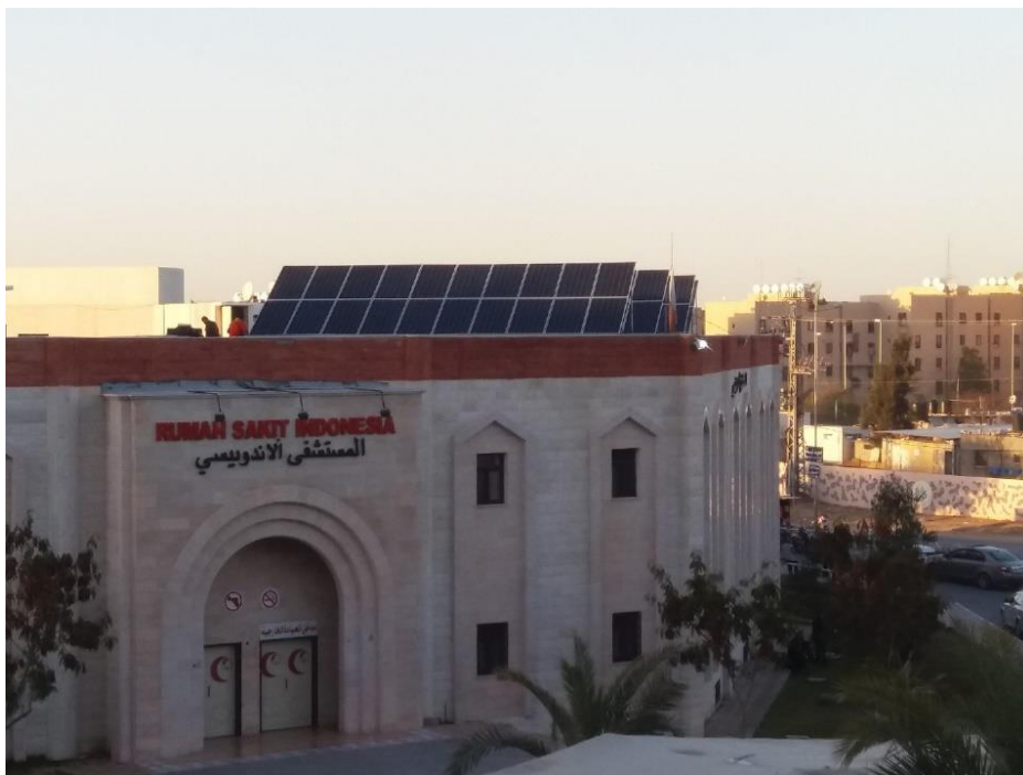
Figure 2: PV Solar Panels on the top of the Indonesian Hospital
