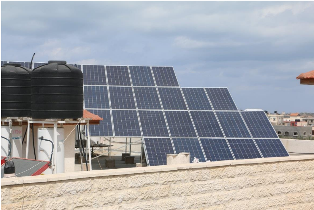
Figure 7: Solar Panels on the top of Al Aqsa Hospital
