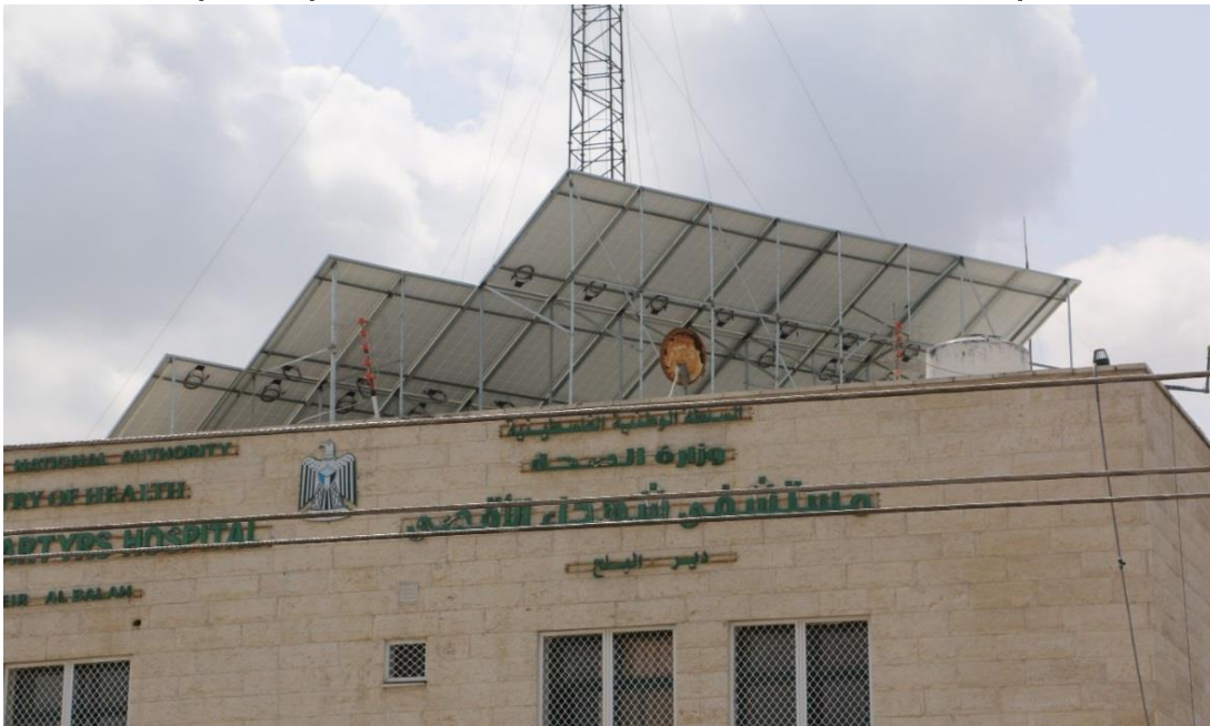
Figure 6: Solar Panels on the top of Al Aqsa Hospital in Deir El Balah
