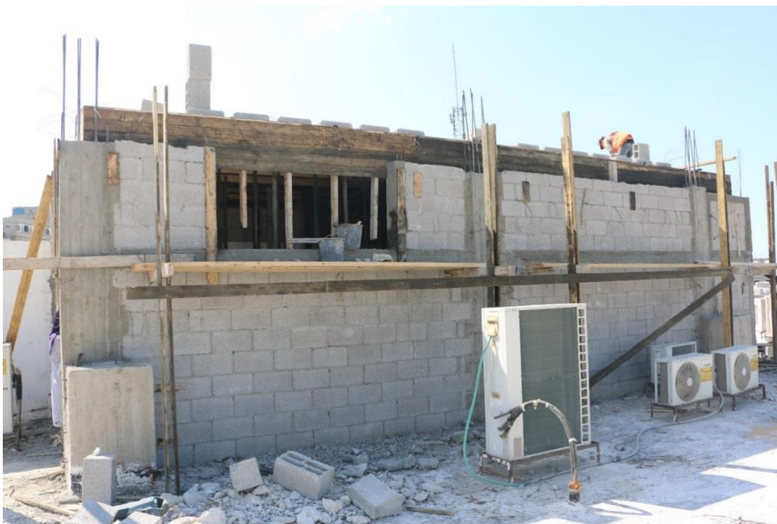
Figure 4: Construction of the Batteries Room on the top of the Indonesian Hospital
